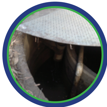
(b) Sludge pit after biological treatment
