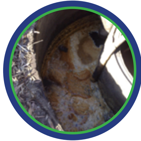
(a) Sludge pit before biological treatment
